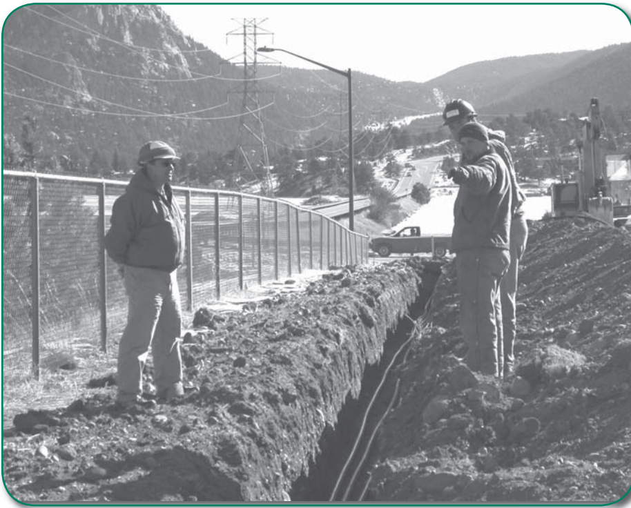
Town employee Mike Mangelsen inspects a trench with Jason Henning of Kearney and Sons Excavating and Cornerstone Engineering's Kerry Prochaska, general contractor for the project at Stanley Park. Undergrounding the electrical service at the fairgrounds is one of the upgrades currently underway at the facility. Mangelsen is project manager for the Stanley Park renovations.
